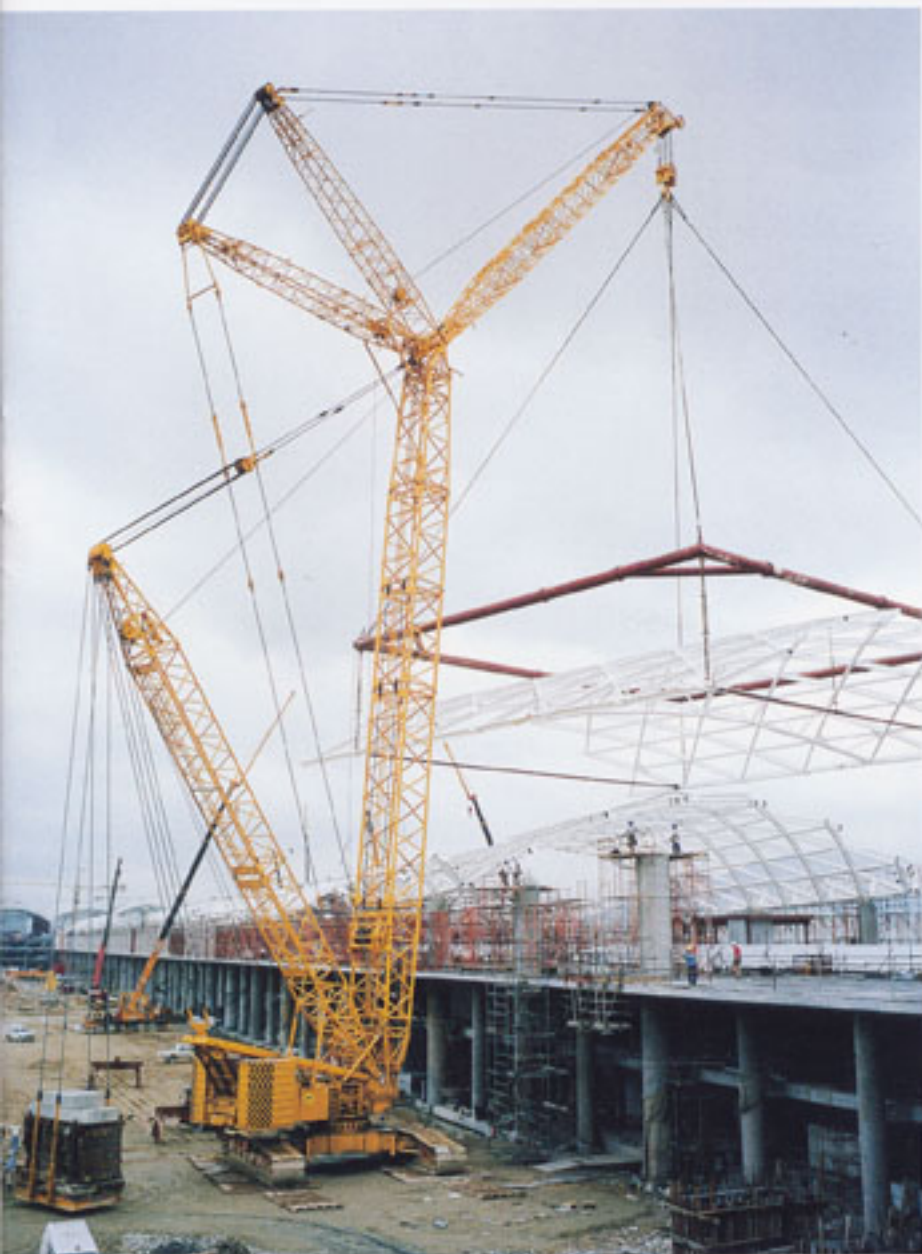
Hong Kong - In April of this year the Check Lap Kok Airport will handle its first commercial flight. The roof of the 1.2 kilometer long passenger terminal complex was assembled modular-wise. Walter Wright Mammoet took care of transport and lifting of a total of 129 roof modules by means of lattice boom cranes of the types CC2600, CC4000 and CC4800. Pictured is the Demag CC4800 positioning one of the roof modules.
